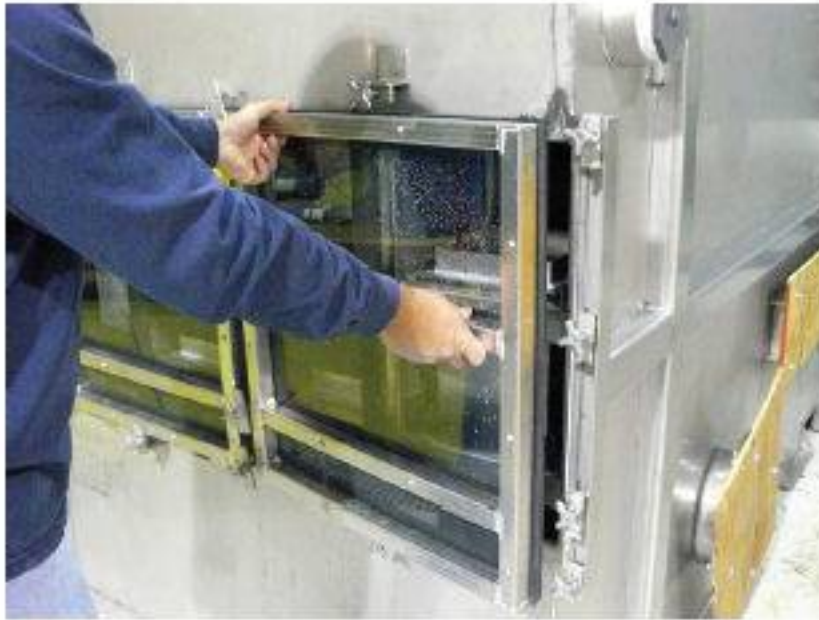
1. Remove access doors / hatches as you normally would to gain access to the internal tray areas of the air stripper.
